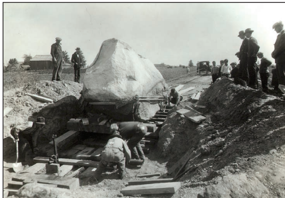
Workers shown removing the 123,000-pound boulder from a Kinde farm field, September, 1929.
