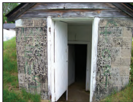
Two wooden doors help control the temperature and humidity.
