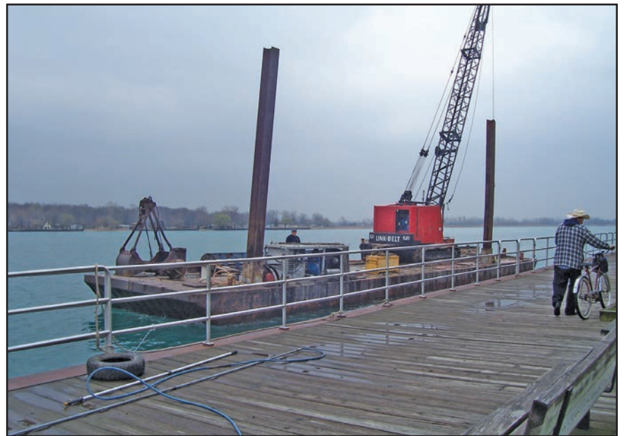
The crane on the barge is used to remove the broken pylon.
