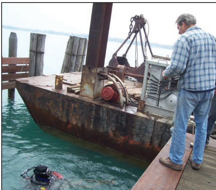
Diver Kodet and Captain Bud coordinate their plans for removing the broken pylon.
