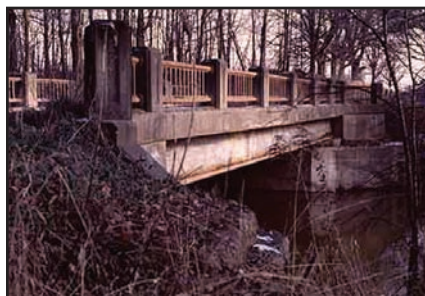
The Masters Road bridge in Riley Township was built during the Great Depression.
